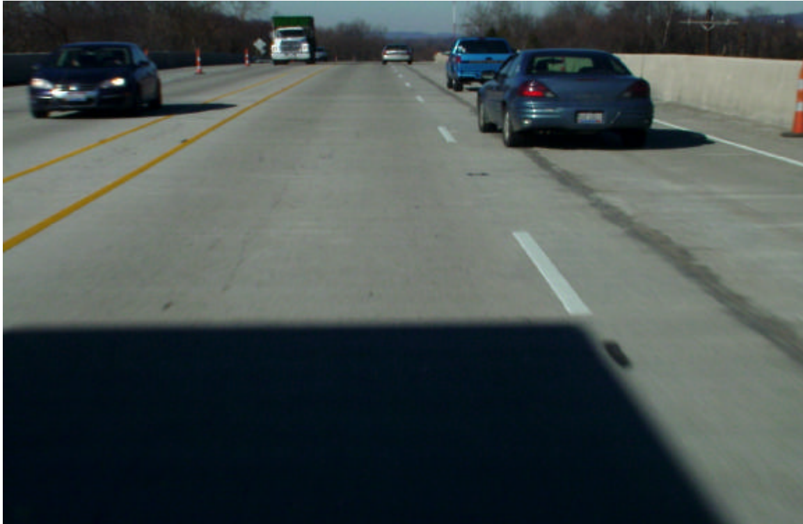
Figure 4. Construction joint in left wheel path of right lane.
