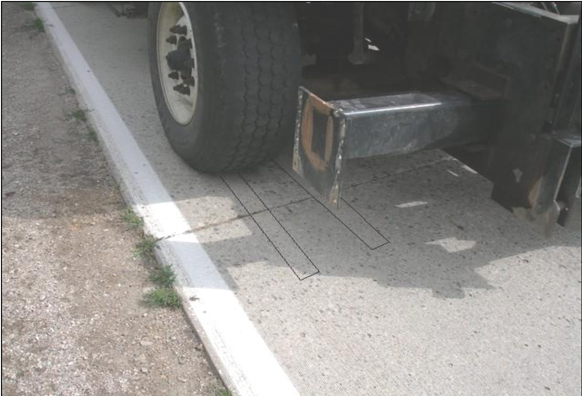
Figure A.13. Truck driving over doweled joint (retrofit trenches outlined)
