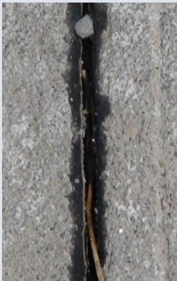
Figure 8 Unsatisfactory Filled Joint
