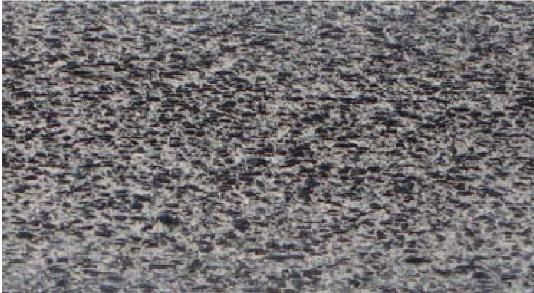
Figure 10: View of the coarse aggregate fins 10 years after grinding, when the gap between the blades was set too wide
