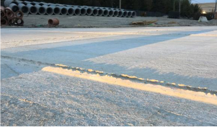
Figure 4 Photo of Concrete Remains from Early Entry Sawing without Vacuuming
