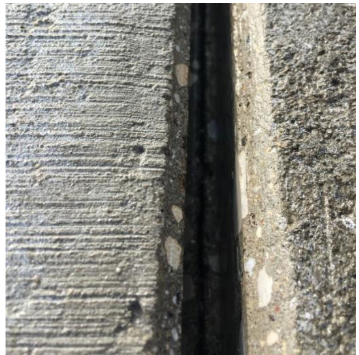
Figure 3 Photo of Wet Saw Joint Condition After Power Washing and Vacuuming
