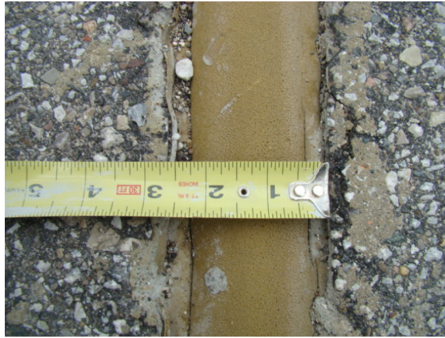
Figure 36. Inspectors should measure the joint to prevent future damage
