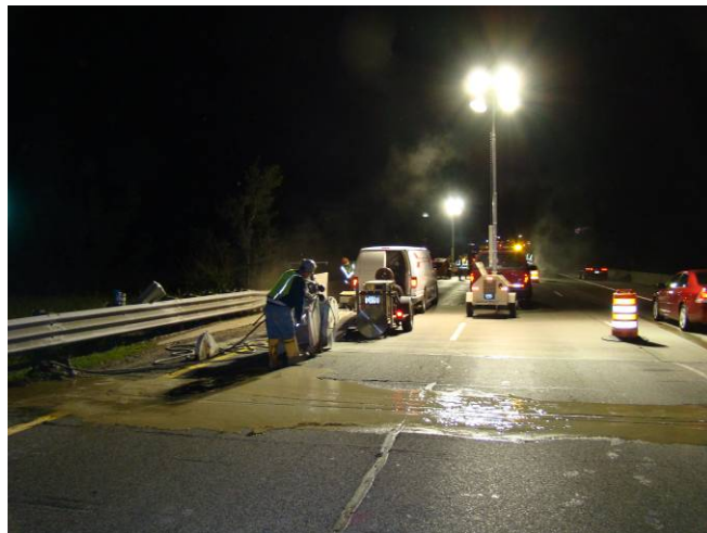
Figure 35. PRJ installations also work well during night time hours
